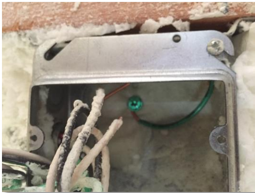
This picture was taken of an electrical box at the Arbor Trails Senior Housing on Blairs Ferry. It shows insulation sprayed into the outlet box, which is a violation of the Electrical code not allowing foreign (non-approved) materials in any electrical installation. The insulation company should have covered them before spraying. Since they didn't they had to go back and clean the combustible material out of each box.
