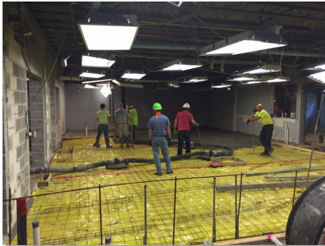
Contractor pumped concrete over 300' to pour the Linn Mar Kitchen floor. You can see the hose laying on the floor.
