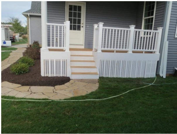
Need hand rail on stairs over 30" in total rise
