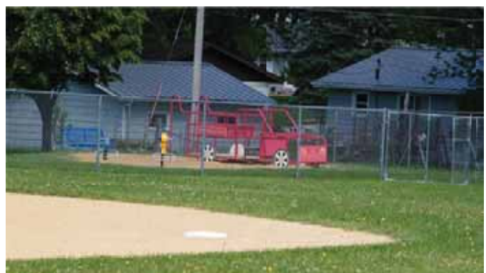
Image 2: The older playground structure is difficult to access and in need of replacement.
