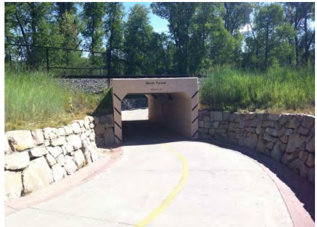
Figure 102: Trail underpasses separate trail users from motor vehicle traffic and/or rail traffic, reducing delays for all users.
