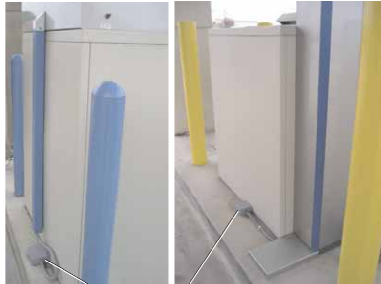
Power is routed externally from a dedicated source separate from the ATM
