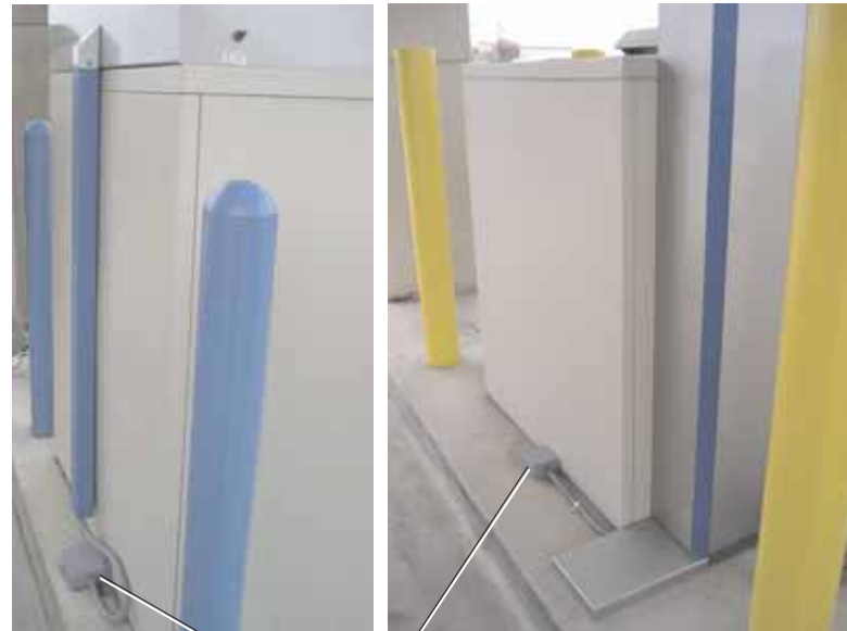
Power is routed externally from a dedicated source separate from the ATM
