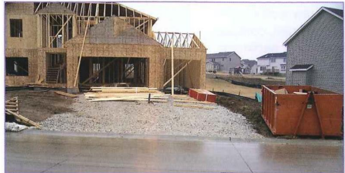
This rock entrance provides mud-free access for construction workers and building materials.
